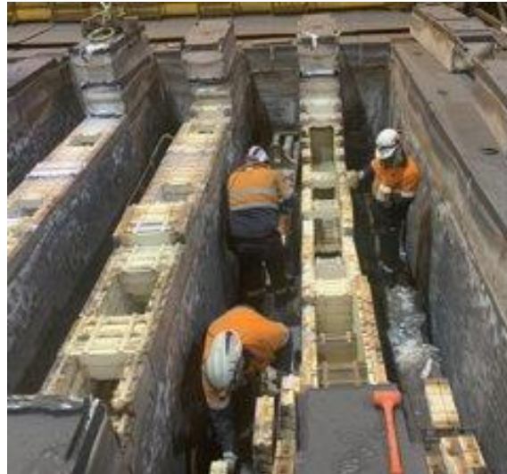
Figure 7. V-shape repairs being carried out to restore pinching below gas injection peepholes.
